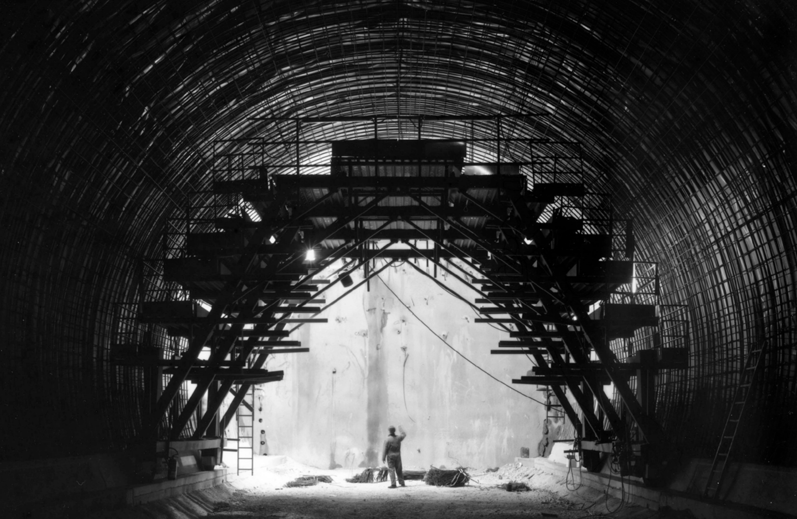
Italy, Cancelli-Vitulano, Naples-Bari Photo by Domingo Milella from the photographic project "Nuove Avventure Sotterranee"
